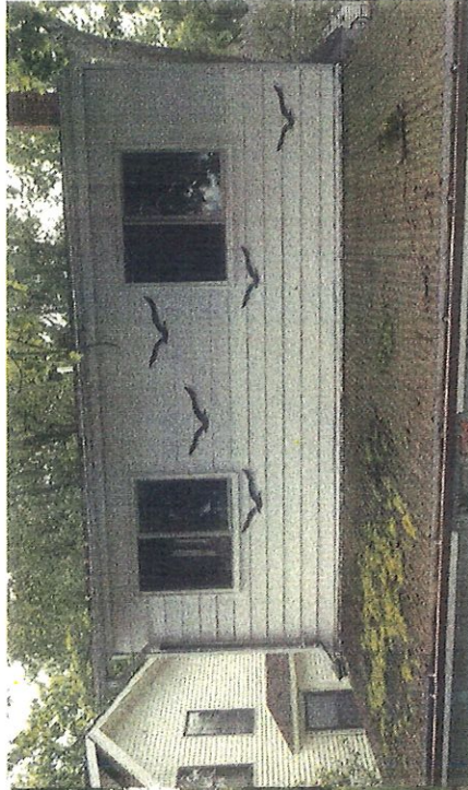
MOLD ON LEAKING ROOF
